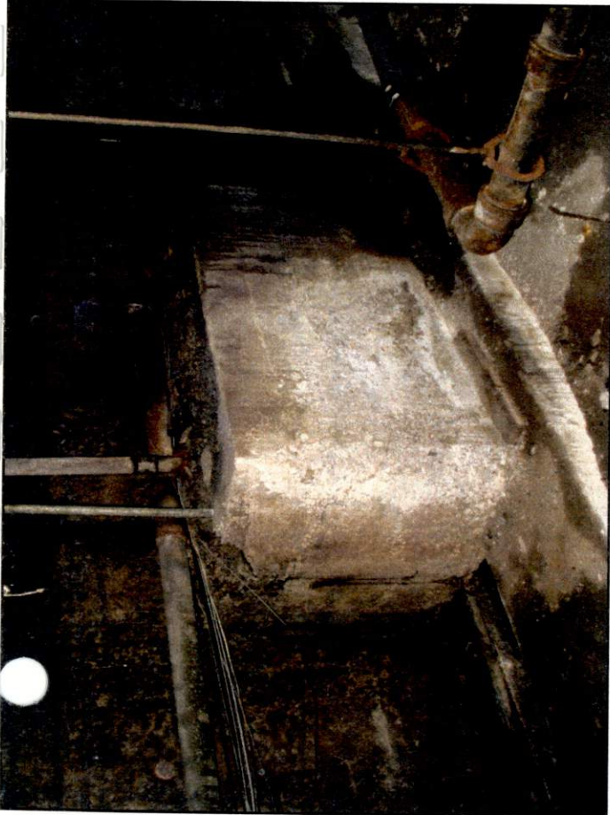
Photograph 5: View of the concrete box and extruding piping located beneath the Exchange Street sidewalk (January 3, 2003).
