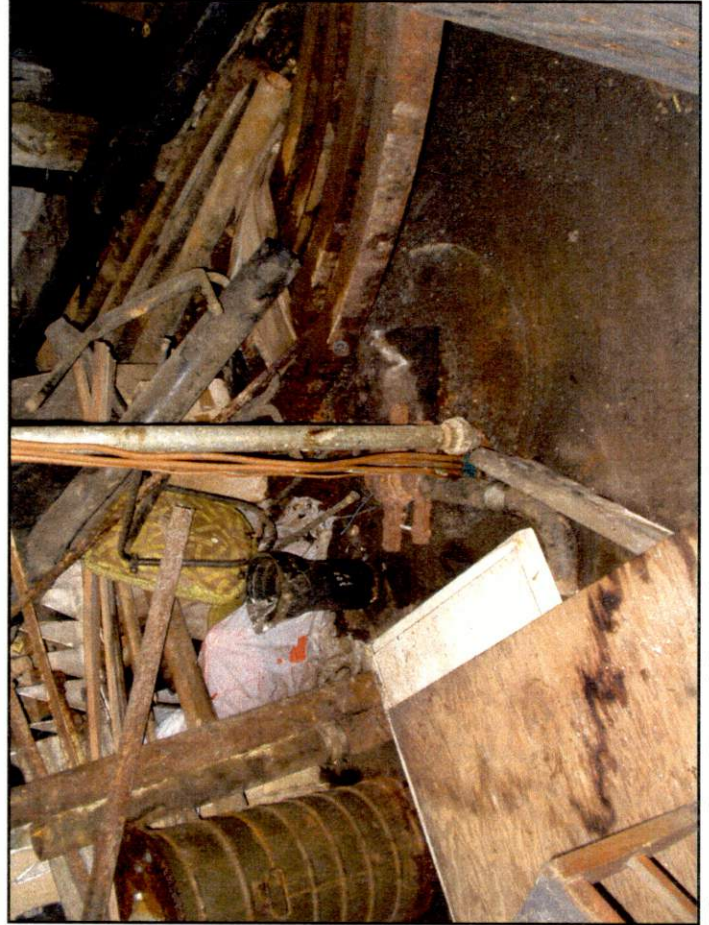
Photograph 3: View of the underground heating oil tank manhole and piping located beneath the Exchange Street sidewalk (January 3, 2003).
