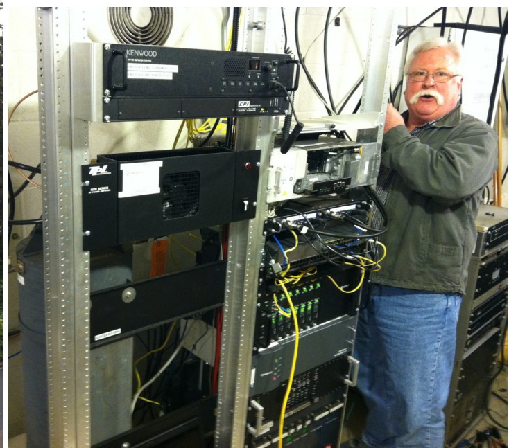
A radio technician from Day Wireless performing maintenance at the Coxcomb Radio site. Part radio, part network site each of these sites grows in complexity.
