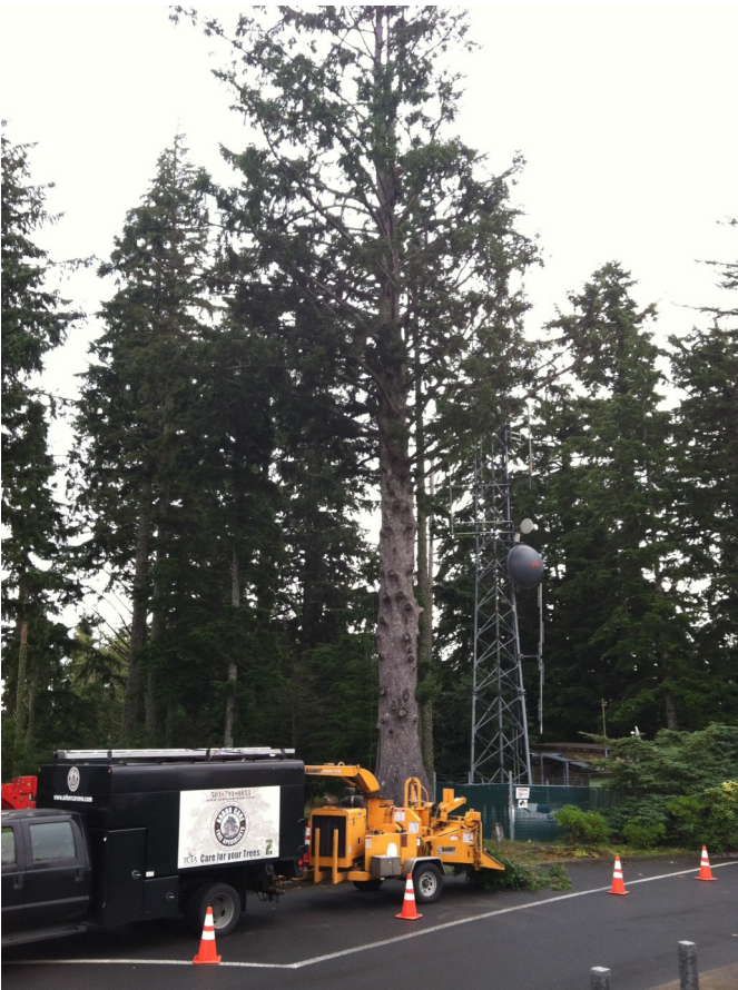
Arbor Care Tree Service working to remove a tree threatening the Coxcomb communications tower.
